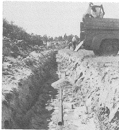
Experimental deep tile drainage line being installed at the Indian River Field Laboratory.
