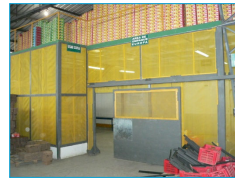
4. Screened treatment area
